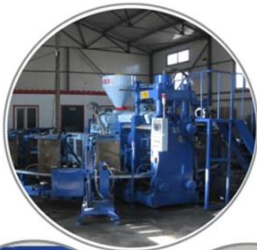
Automatic Injection Molding Machine
